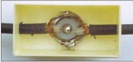
Figure 14: Junction box for a group of two
